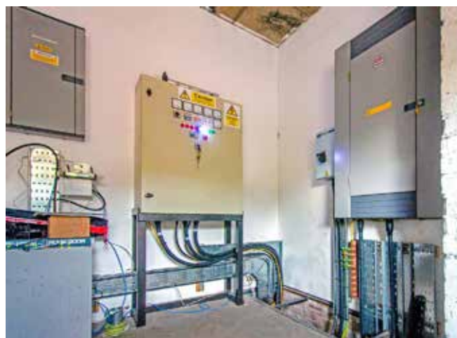
Incomer room. We cleaned and lined this room, digging out all the ducts, pulling in plastic liners and fitting cable trays. This picture shows the bunker being supplied on-load from the generator. The panel in the centre is the generator control panel and the power change-over unit. The panel on the right is the master distribution panel with circuits for each of the building areas. The power supply company switchgear for the permanent 3-phase supply will be fitted to the left of the master distribution panel
